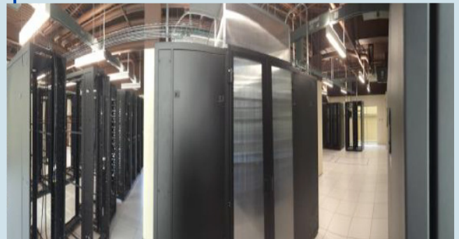
Figure 15: The layout of the data center lab. Practical measurements were made and checked against a CFD model. The highly accurate results led to ES2 and Binghamton adopting 6SigmaDCX for future DC operations.
